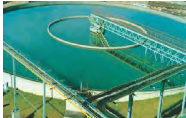
Waste water treatment plant
