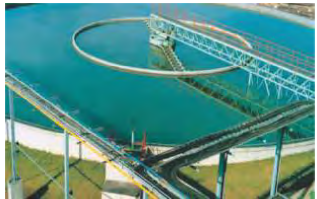
Waste water treatment plant
