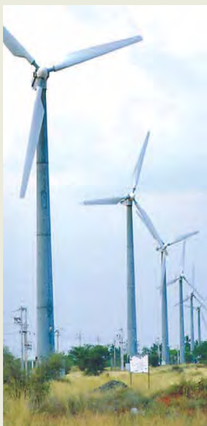
Devarkulam Windfarm (250KW WEGs)
