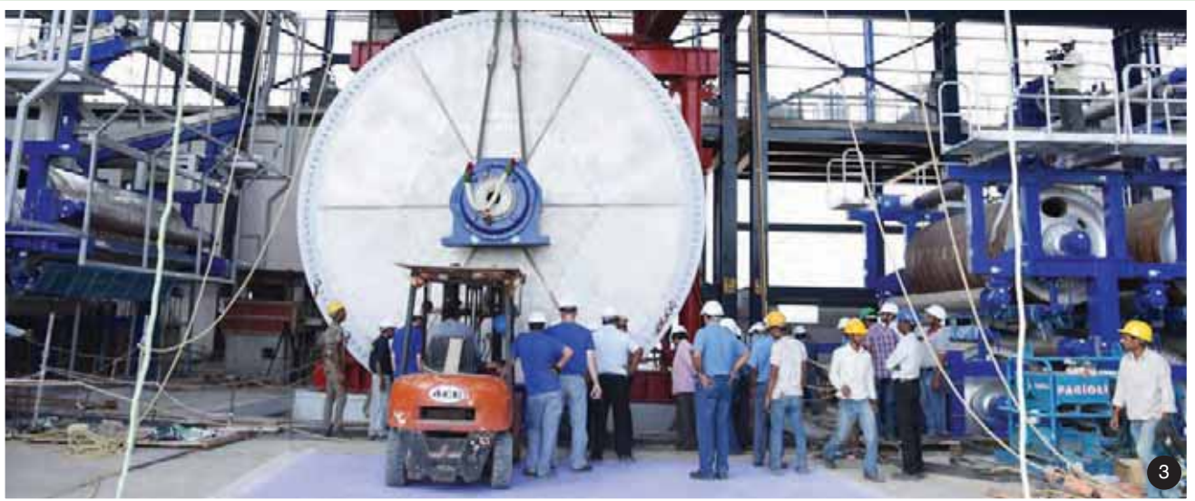
New Board Machine being installed in Mondipatti Village, Manaparai Taluk, Trichy District: (1) Wire Section (2) Dryer Section (3) MG Cylinder
