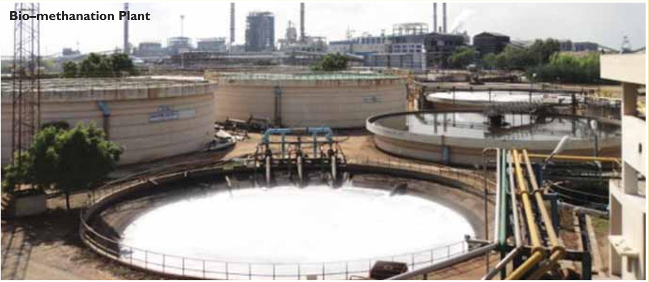
A Modern Waste Water Treatment Plant – Unit-II
