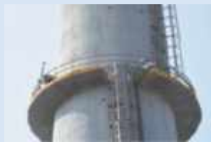
Continuous Stack Emission Monitoring Stations
