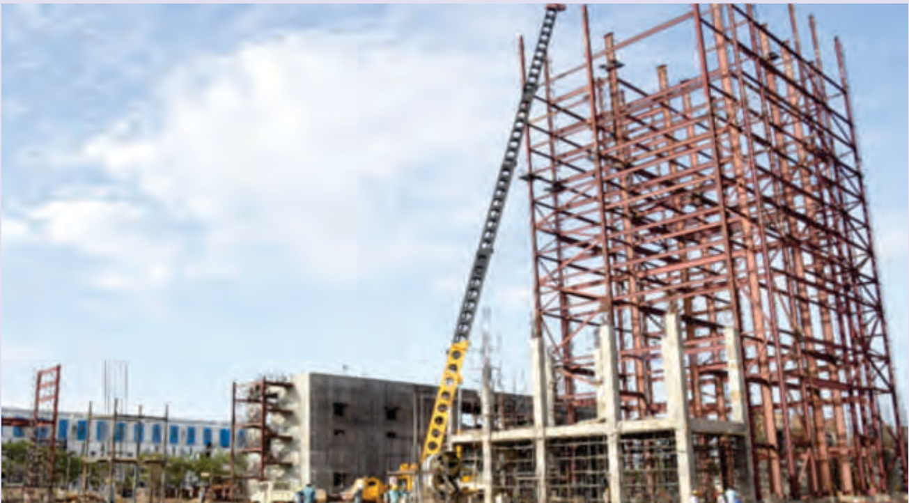
Mill Expansion Plan of Unit II - Erection of Chemical Recovery Boiler in progress
